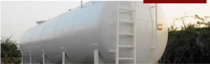
Fixed Diesel Tanks
