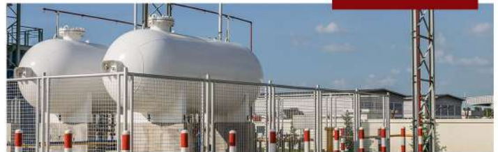
Compressed industrial gas Storage System.
