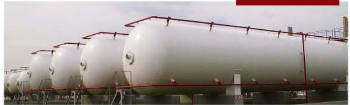
New/Existing LPG system
